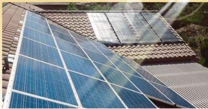
Many Malaysians have installed solar panels at home.
