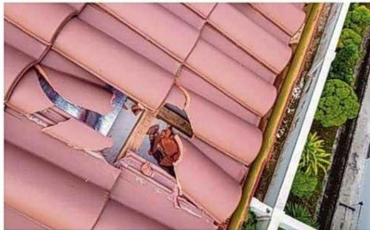
Blasting at a quarry in Sungai Ara, Bayan Lepas, is believed to have sent rocks hurtling into a residential area nearby.
