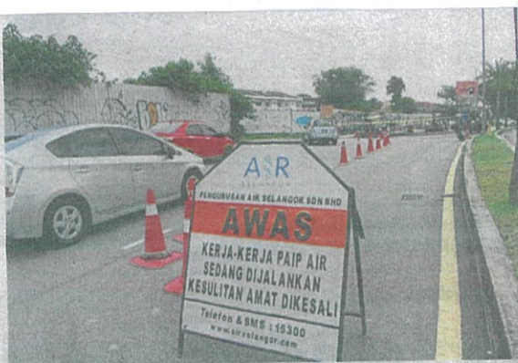
Part of Jalan Universiti, Petaling Jaya was closed to motorists following a burst pipe incident on Wednesday.
