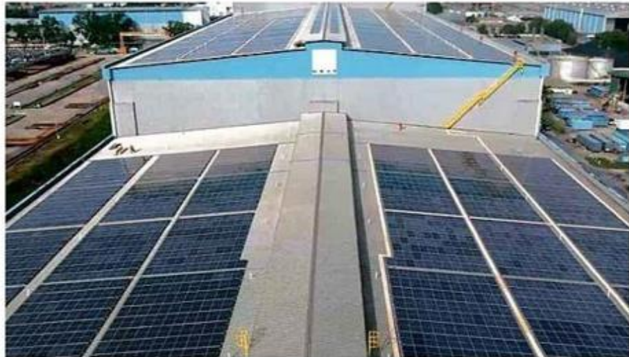
The rooftop solar system installation at Malaysia Marine and Heavy Engineering Holdings Bhd's premises in Pasir Gudang, Johor, or MMHE West, can produce 8.33MWp of power.
