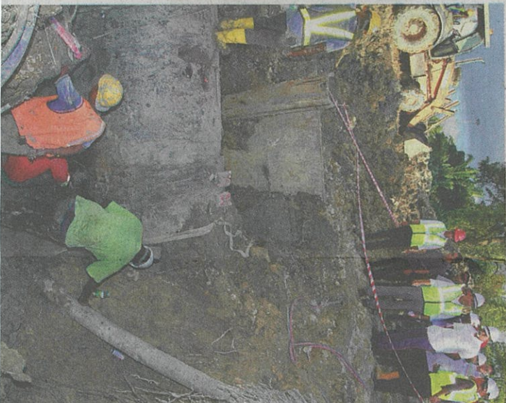
Repair in progress: Dr Xavier visiting the site of the ruptured pipes in Klang.
