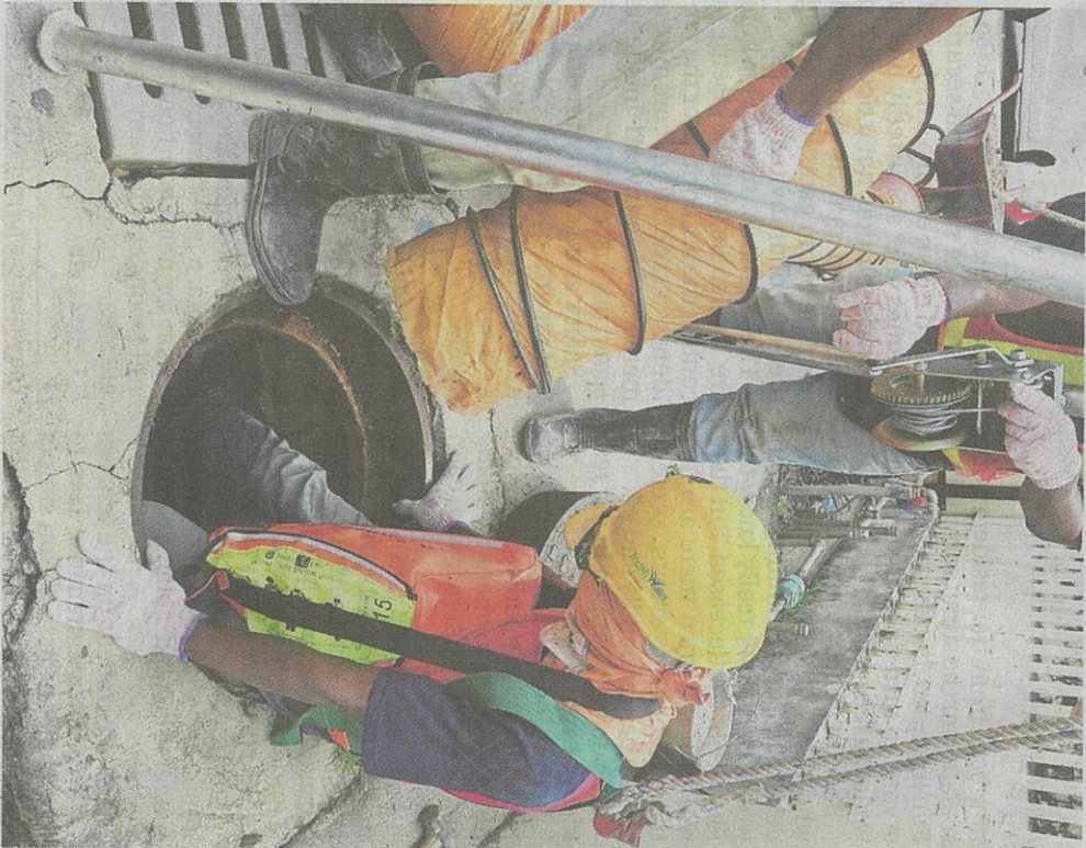
Indah Water Consortium workers descending into a sewerage shaft to disconnect sewerage services.
