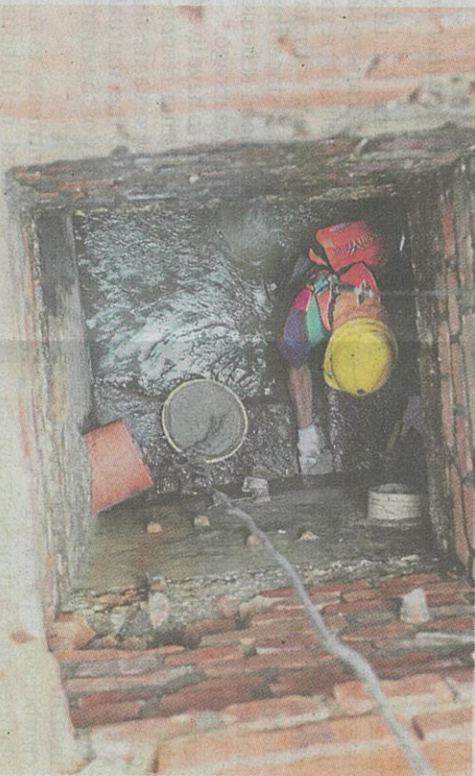
A worker sealing sewerage pipes that are connected to the errant customer's premises. This is done by using cemented bricks and it does not disrupt the sewerage services of nearby premises.
