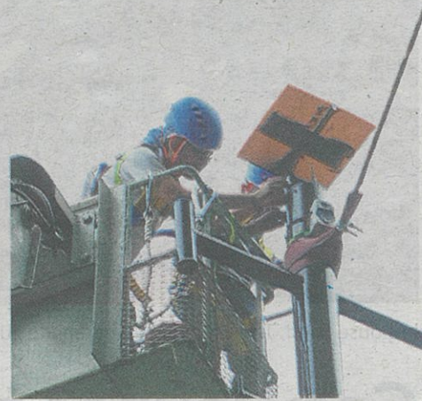
Volunteers building Malaysia's first urban wildlife canopy bridge along the busy coastal road of Teluk Bahang, to help primates cross roads safely.
