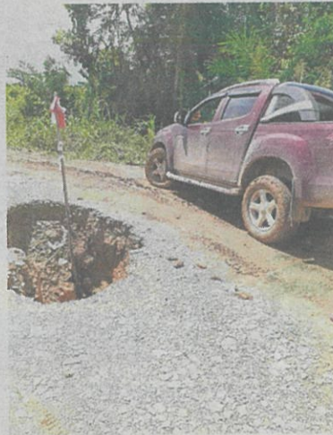
Cause for concern: A hole in a rural road leading to Long Ikgang in northern Sarawak.
