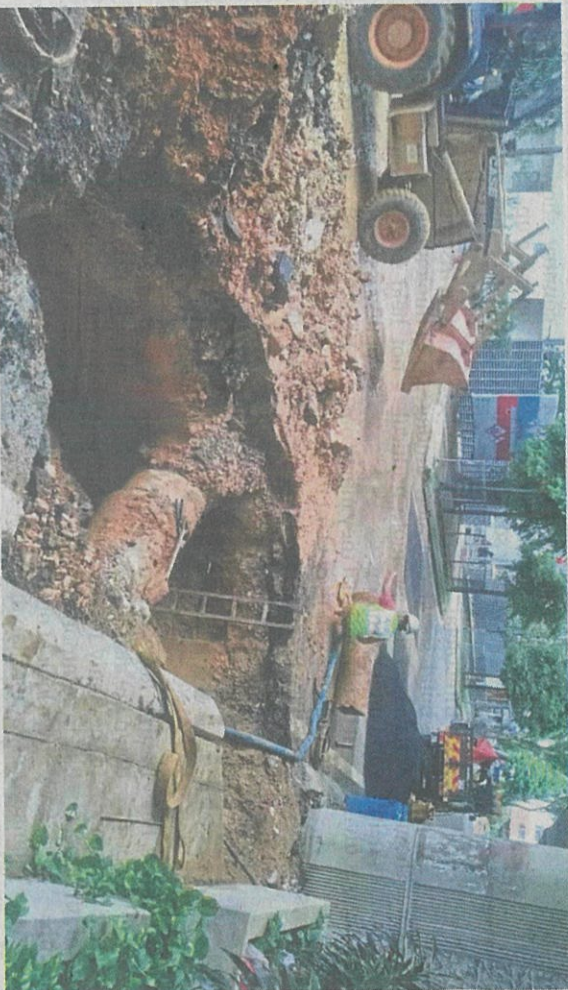
Work in progress: Syabas personnel repairing the burst underground pipe along Jalan Dewan Bahasa in Kuala Lumpur.
