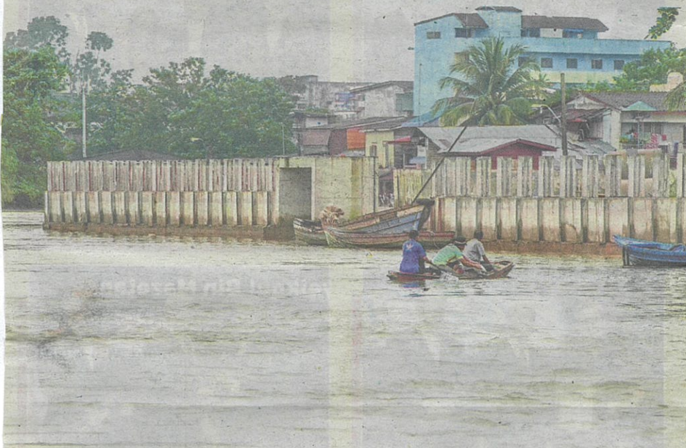
Cause for concern: The cement wall being built by the Thai government on the Malaysia-Thailand border near Rantau Panjang. — Bernama
